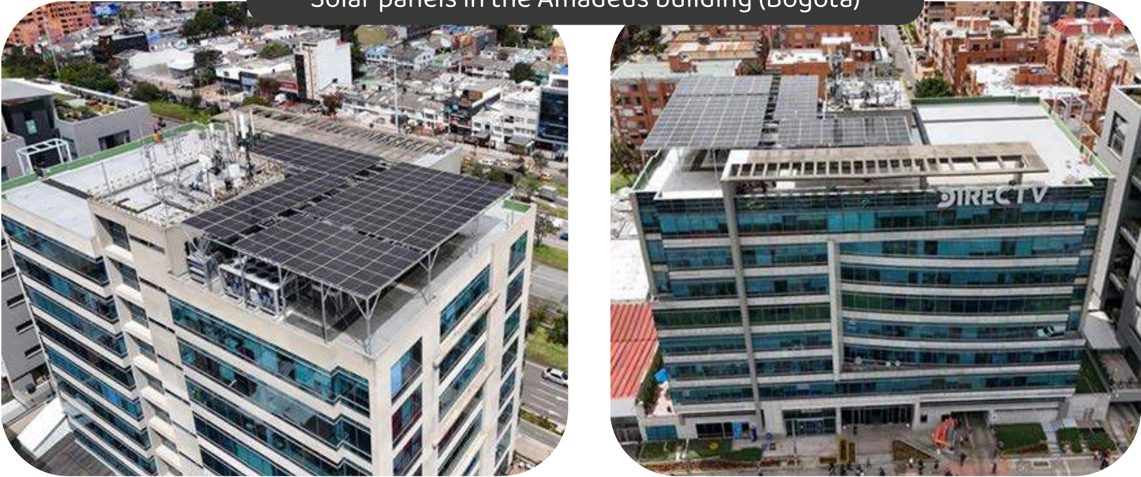
Solar panels in the Amadeus building (Bogota)
